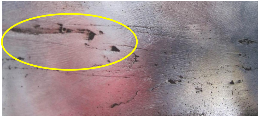
Photo of pipe joint - Anomalies 2148 and 2149
