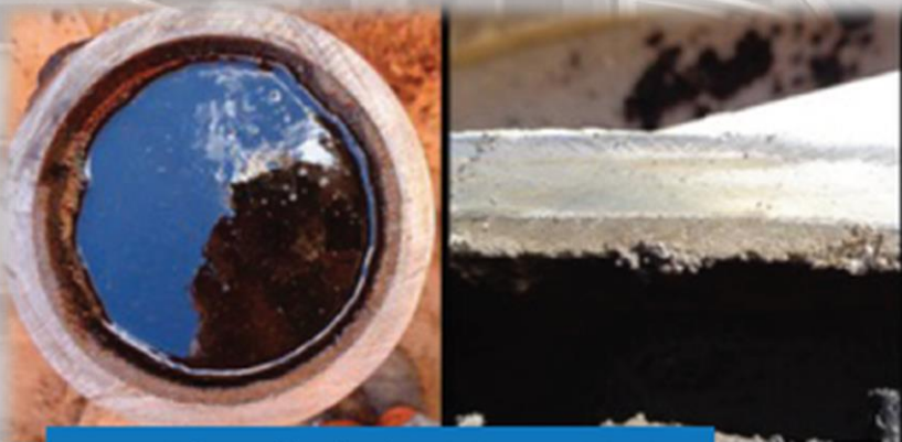
Volume of hard sediment remaining in a 6" crude line measured and mapped by GEO+
