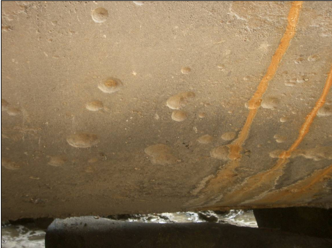
Figure 7 Multiple Deep Pits
