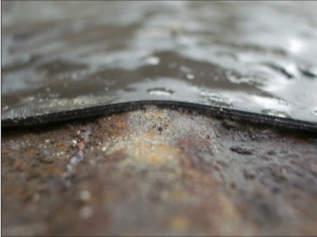
Figure 6 'Tenting' Of A Tape Wrap Coating
