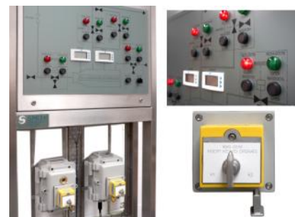
Smith Flow Control's custom-built operating panel
