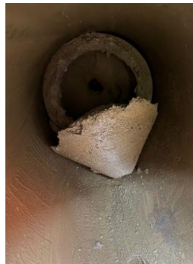
Damaged foam pig
